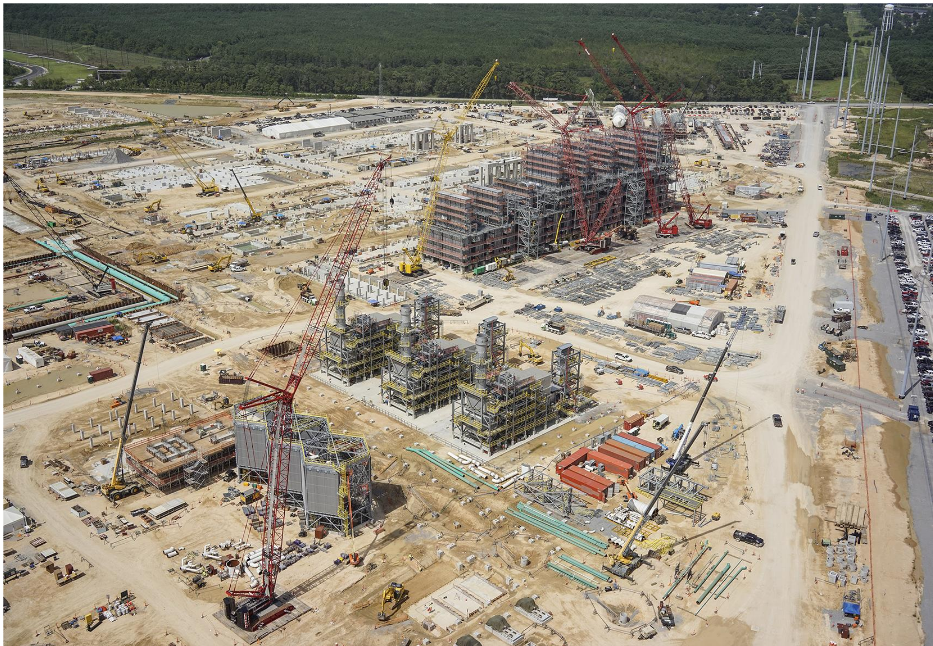
Cracker furnaces installed, LCCP, USA
