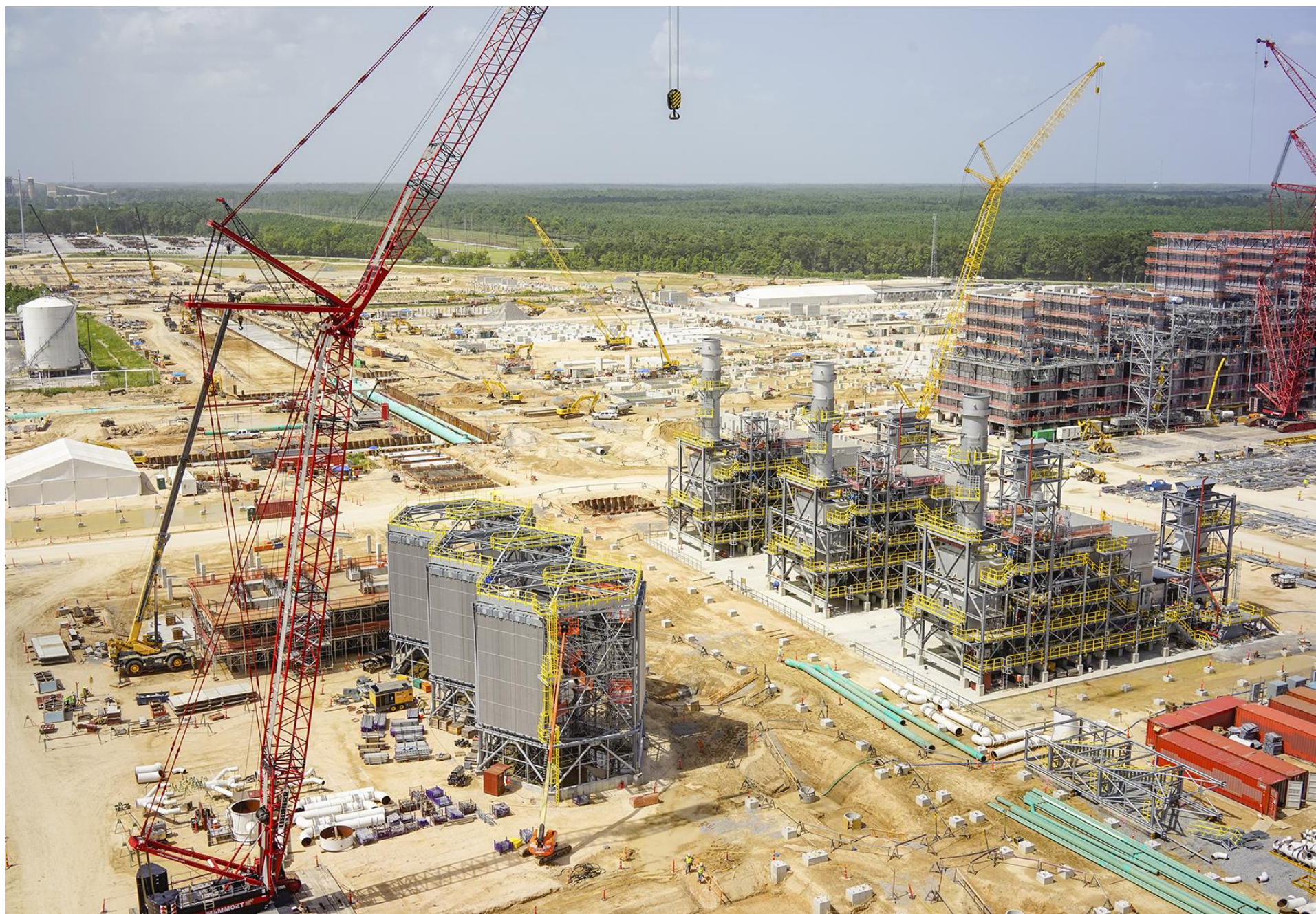
Three boilers installed at site, LCCP, USA
