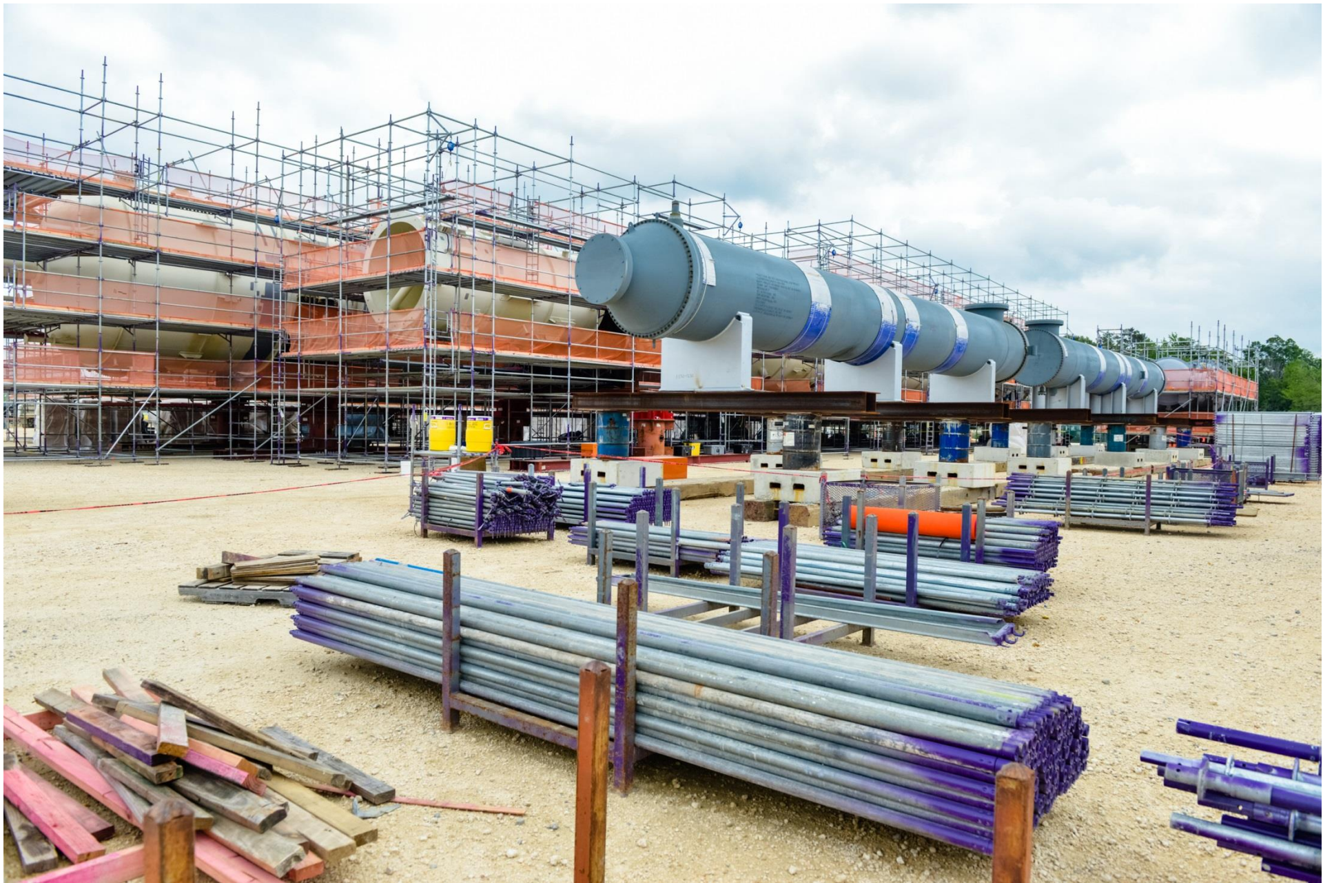
Cracker tower dress-out, LCCP, USA
